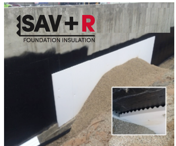
Figure A SAV+R installed on a foundation wall
